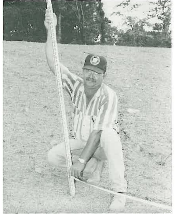
Doug Smith , Construction Aide III for District 6, checks grades along a new section of Highway 270 in Hot Springs.
