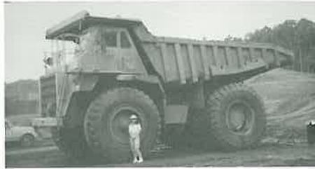
Stacye Roam, Field Clerk II in the Alma Residency, stands next to a "large" dump truck being used on the Highway 71 relocation project near Mountainburg.
