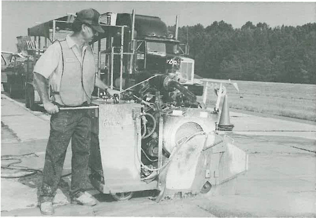
Kenneth Jones , Bridge Repairer II on the District 8 bridge crew, operates a concrete saw in preparation for concrete patching along a section of Interstate 40 west of Conway.
